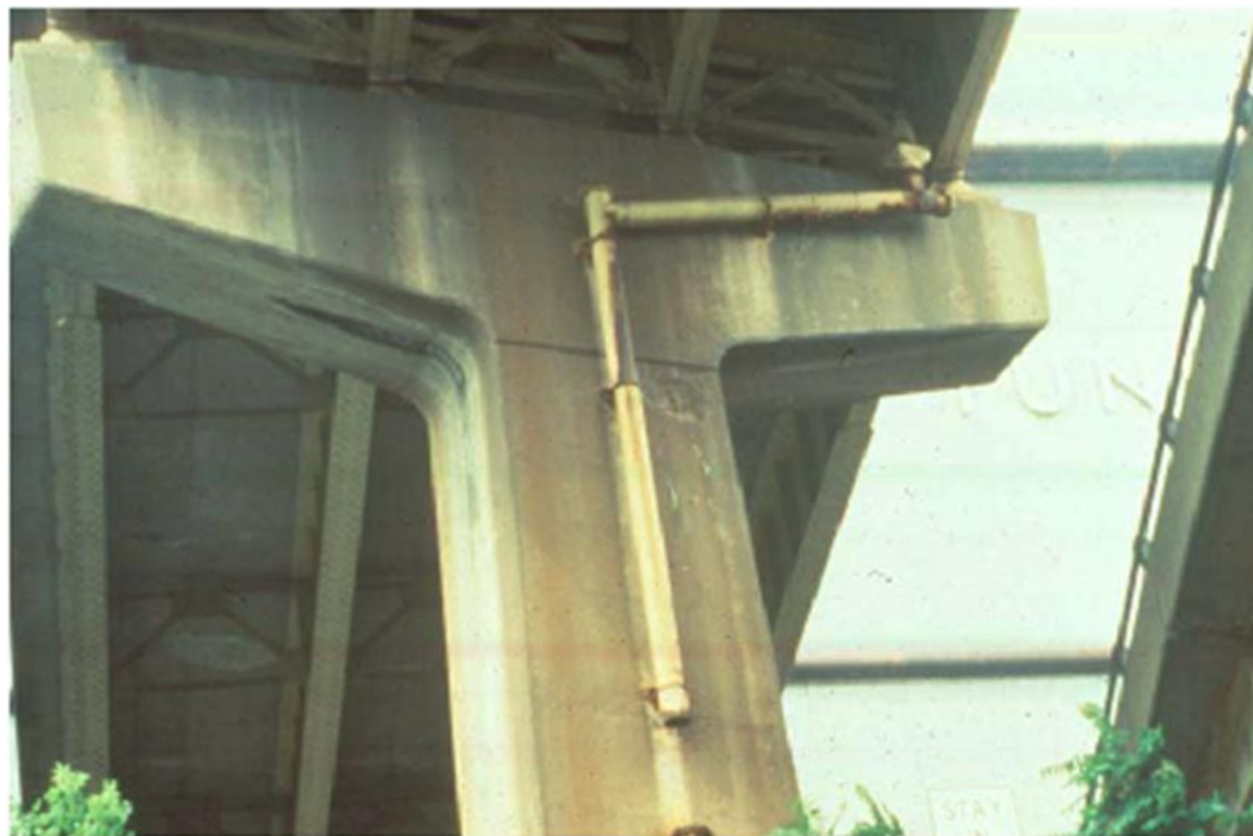
Figure 5.4.14 Downspout Pipe and Cleanout Plug
